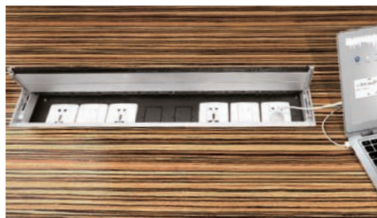
会议桌线盒打开状态 Opening state of conference table line box
